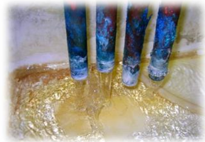
Figure 8: discharge pipes from mains-to-drain cooling in the Physical Chemistry Building
